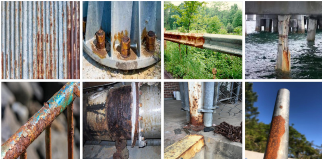
Figure 4. Examples of 1st dataset images highlighting corrosion on different metal structures and surfaces [12].
